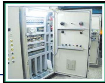
Field Control Panel
