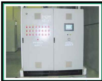
Master Control Panel
