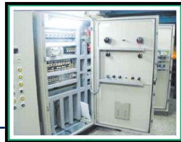
Field Control Panel
