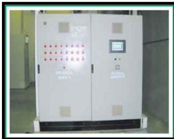
Master Control Panel
